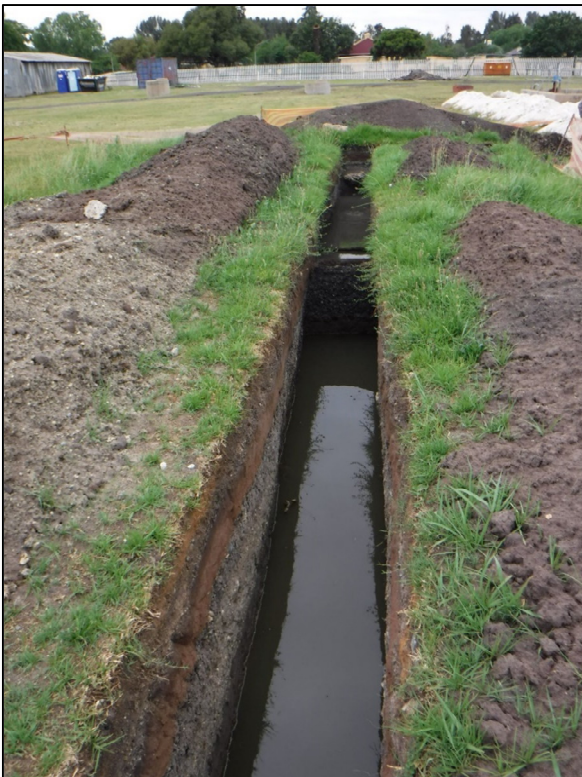
Plate 4. View of typical trench excavation on site, which is partially filled with water.
